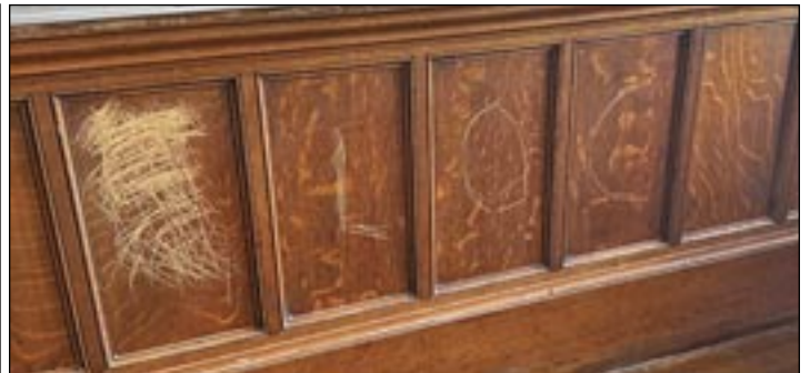
Woodwork in one of the historic classrooms of Fairhaven High School is scratched and carved up after vandals broke into the building on 5/16/26. Photo courtesy of the Fairhaven School Dept.
