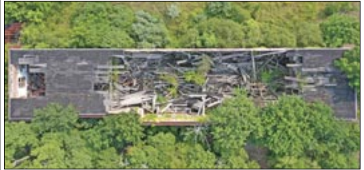
An aerial photo from July, 2025, shows the extent of the collapse of the roof of the Atlas Tack building in Fairhaven, a superfund site that has been neglected for years. Photo courtesy of the Town of Fairhaven.
