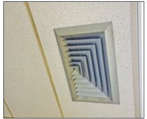
AFTER photo: the ceiling tiles are replaced around the vent in the basement of St. Mary's Church in Fairhaven on 5/31/25 for the Eagle Scout project of Patrick Fleming from Troop 52. Submitted photo.
