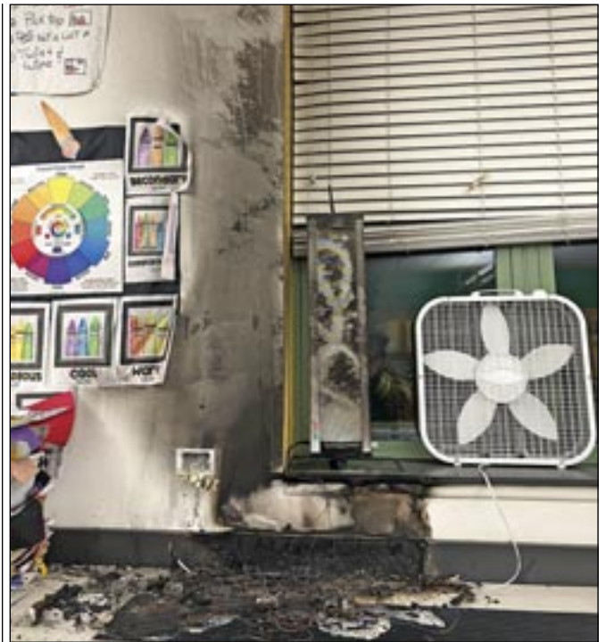
The Fairhaven Fire Department believes the fire at East Fairhaven School on 9/22/24 started in this outlet powering a fan, causing minimal fire damage, and enough smoke damage to close the school for at least three days. Photo courtesy of the Fairhaven Fire Department.
