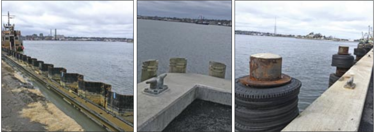
LEFT: The “sheets” that form the frame of the wall at Union Wharf in Fairhaven are 50 feet long, with most of that length driven into the bottom. The i-beam holds the sheets together. Next will come concrete. MIDDLE & RIGHT: The bulkhead on the southwest corner (middle) and on the west side (right) have been rebuilt and show what the north side will look like when finished. Photos by Beth David.
