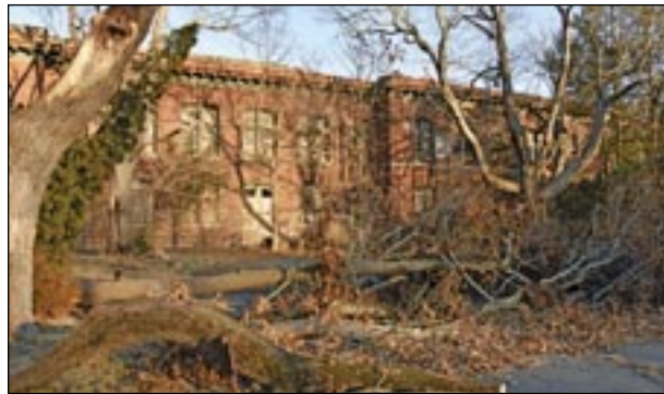
The Atlas Tack building sits abandoned and slowly deteriorating on 1/24/22, a hazardous waste site that the town wants to remediate, making it onto the list of objectives during the Fairhaven Select Board's goals and objectives meeting on 1/22/22. Photo by Beth David.
