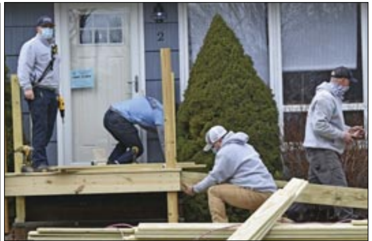
ABOVE: Members of the Fairhaven Firefighters Union, Local 1555, build a ramp on 3/17/21 at a house in Fairhaven to help out a family with a child who is wheelchair bound. L-R: Lt. Josh Benoit, FF/Paramedic Timothy DesRoches, FF/Paramedic Kevin Gonsalves, Lt. Paul Correia. BELOW LEFT: Lt. Correia and Mr. Gonsalves cut a notch in a board for the ramp. Photos by Beth David.
