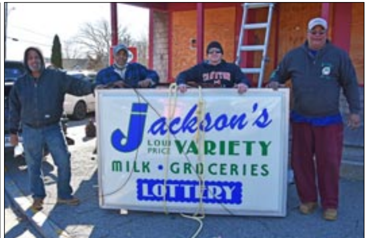
L-R: Peter Collins, Clyde Andrews, Ian Comerford, and Mark Andrews pose with the iconic Jackson's Variety store sign after removing it from the building on Saturday, 2/6/21, one year after fire destroyed the business and severely damaged the building on 2/3/20. Photo by Beth David.
