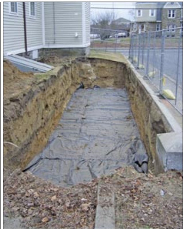
In this January 26, 2021 photo the excavation is mostly complete for the wheelchair ramp and entrance being constructed at the Fairhaven Academy Building, which is home to the visitors center and historical exhibits. Photo by Office of Tourism Director Chris Richard.
