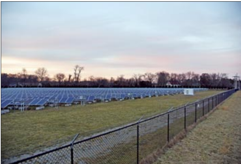
ABOVE & TOP: The Rockett Solar, LLC, array on Wing Lane in Acushnet has been acquired by CVE North America, an independent renewable energy producer based in New York, and a subsidiary of the international company, CVE Group. Photos by Glenn C. Silva.
