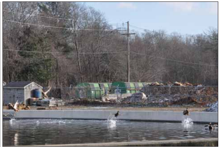
Some ducks are scared away from the tank that is the final phase of treatment for water at Fairhaven's Wastewater Treatment Plant. The water is so clean by the time it is discharged into the bay, that the ducks see no problem with hanging out in it. Photo by Beth David.
