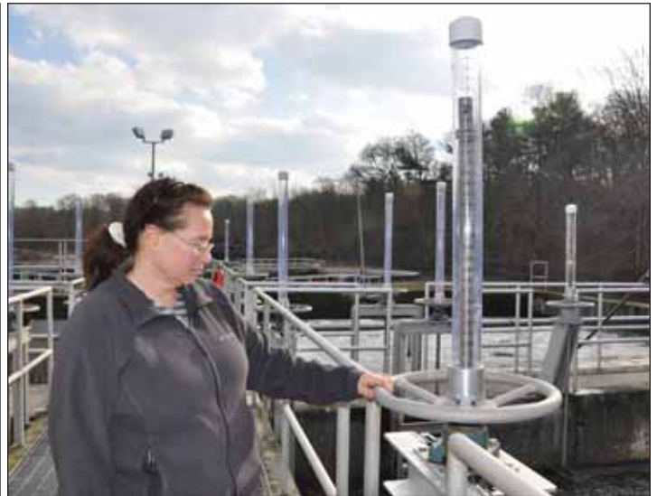
Linda Schick, the sewer/wastewater superintendent in Fairhaven, points out a new gauge that measures oxygen content in large tanks that have to be aerated. Photo by Beth David.
